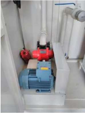
Tank Filling Pump
